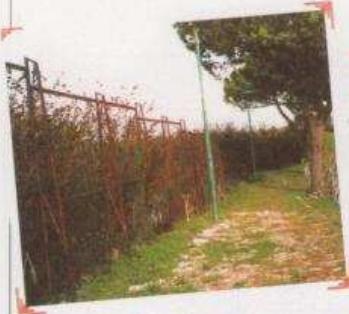
◀ The rusty northern perimeter fence
