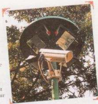
▲ High poles support lighting fixtures and CCTV cameras, some equipped with motion detection capability
